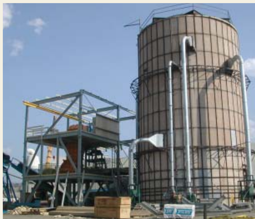
The silo burner at Tolko's Lavington Planer Division, once heralded for its use of leading edge technology, will now rest idly as the new hog processor (left) and conveyor system allows wood production waste to be sent to a co-generation plant in Kettle Falls, Washington.
