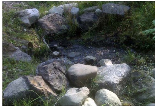
Criterion 3, Element 3.2: Water Quality and Quantity. Culvert outlets have been well armored to reduce potential sedimentation to streams.
